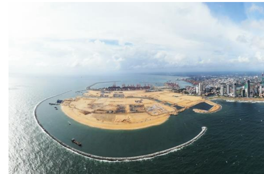
Colombo Port City Project- 2020 ENR Global Best Project Award for Airport / Port Category
